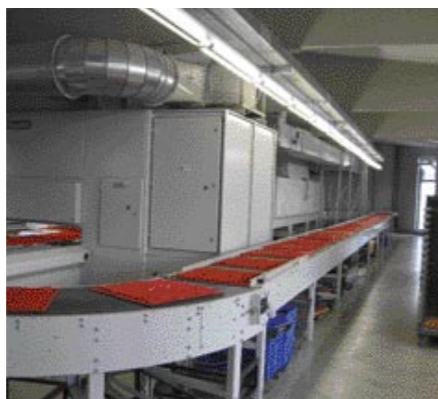
Once the parts have passed through the drying ovens, they are turned over so that every part is fully painted.
